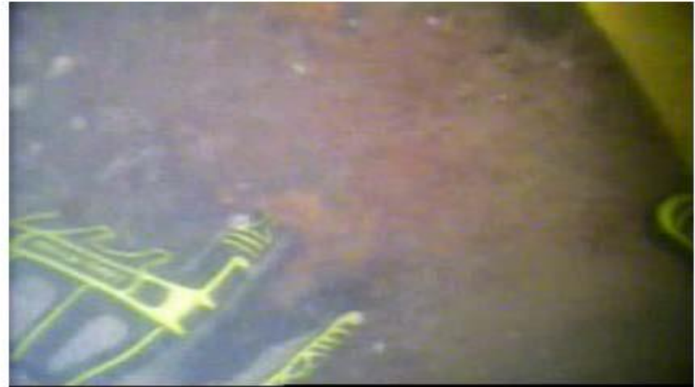
Penetration in Bow Area
