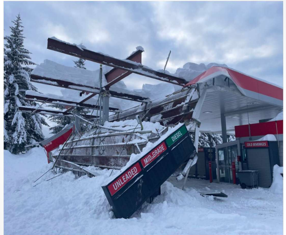
Photos by Mari Kanagy/Juneau Empire The Fred Meyer gas station roof collapsed early morning on Thursday, Jan. 1.
