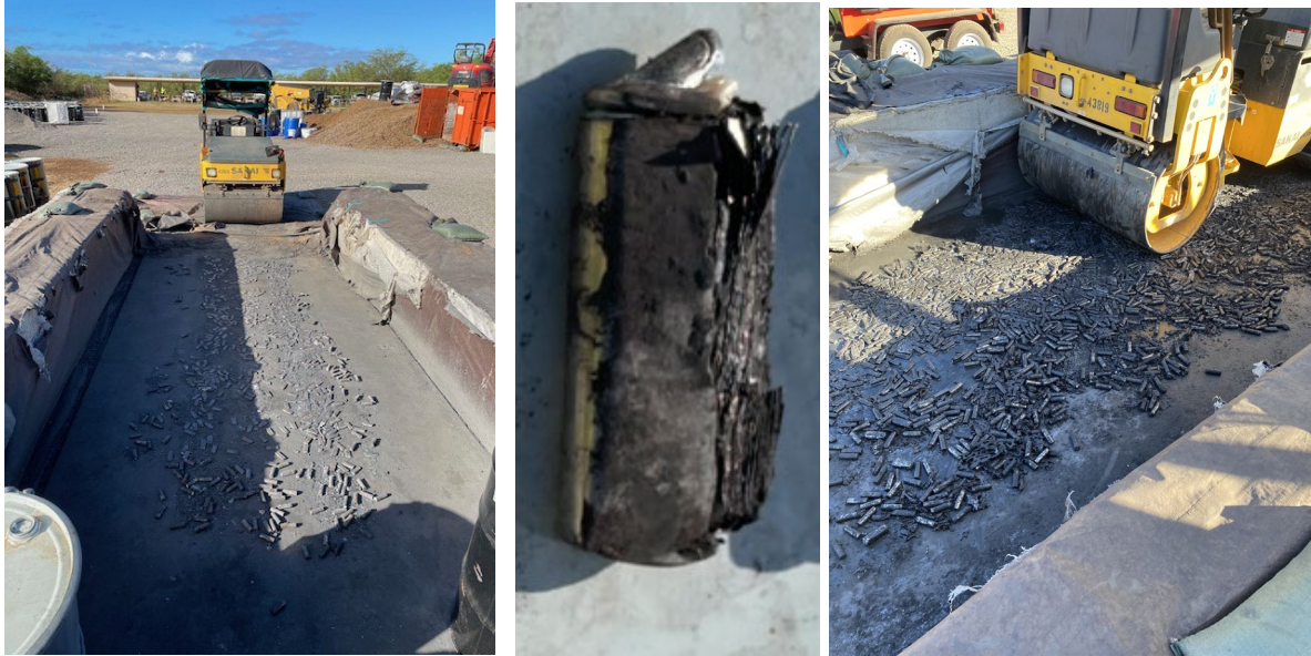
Figure 14: Using a drum roller to crush cylindrical batteries (left and right) and get to a final product for disposal (center).
