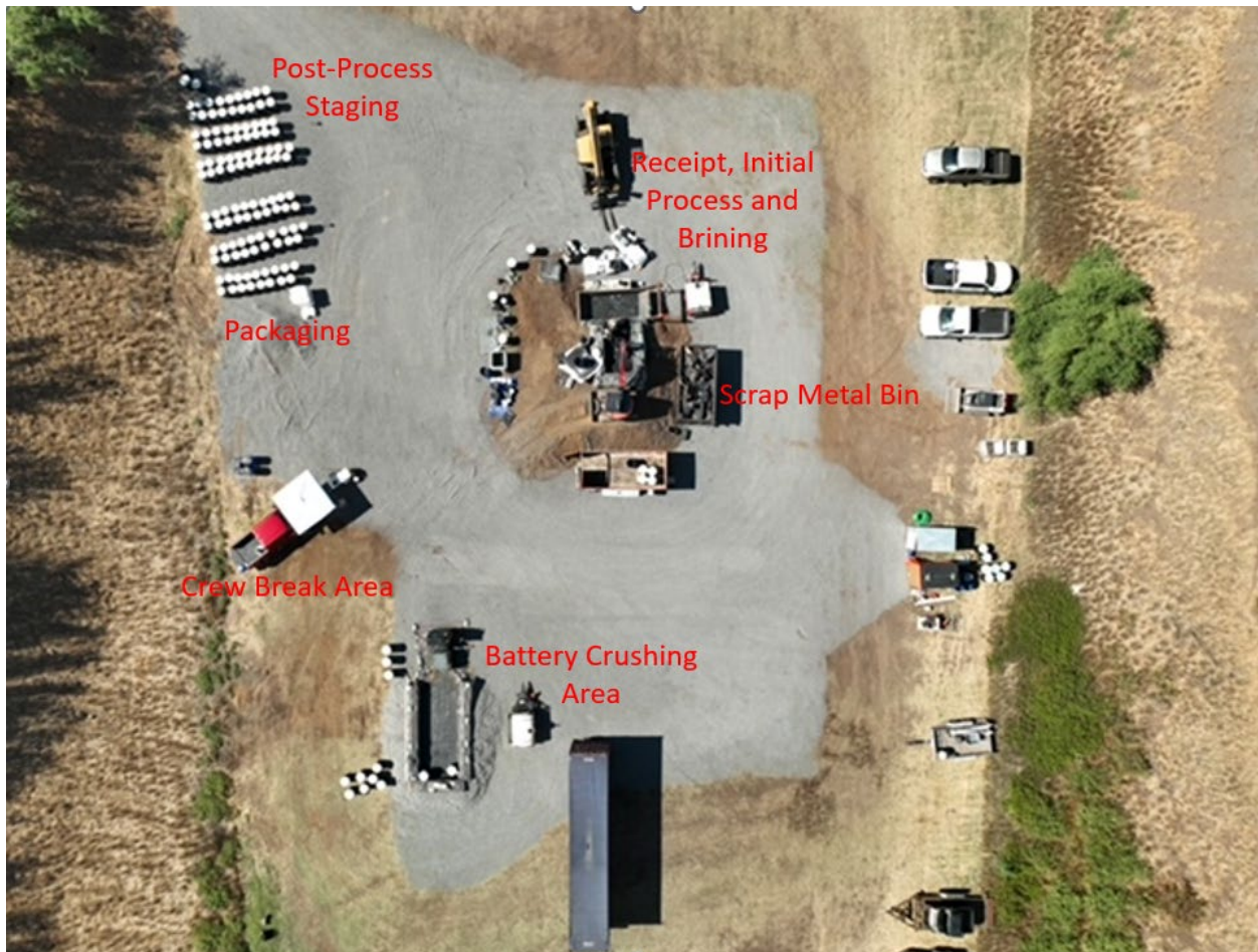
Figure 10: Example of a lithium-ion battery staging area with processing area, de-energizing baths/brining, battery crusher, staging and packaging areas.
