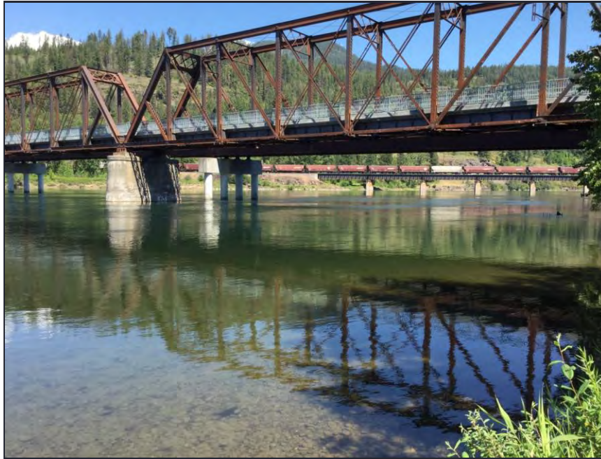
View looking upstream from collection point to River right bridge piling anchor.
