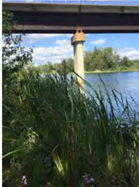
Picture taken from culvert facing upstream, rail link bridge in background for orientation.
