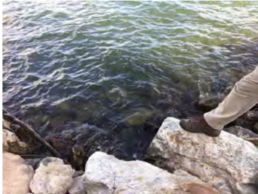
View of culvert. Currently underwater, but fluctuates with lake level from dam use.
