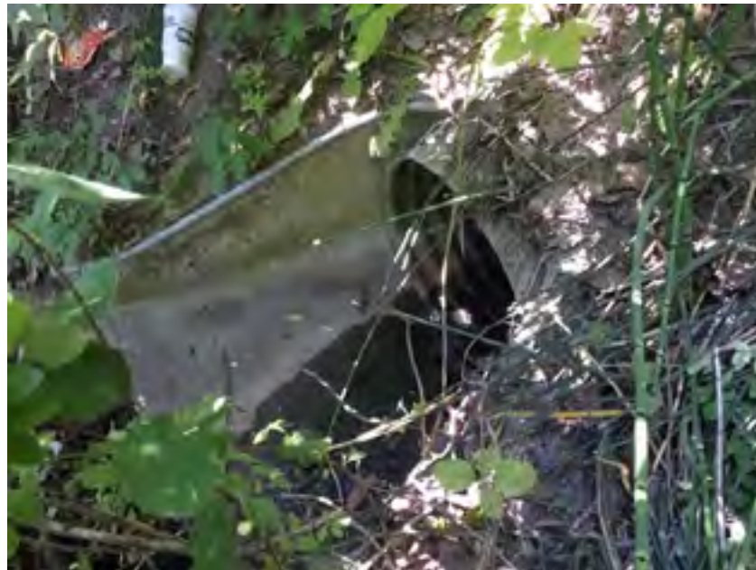
Concrete culvert on shoreline of river, but still difficult to access from water. Closest to Visitor Center.
