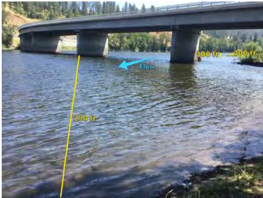
Looking upstream towards midstream bridge pier anchor and upstream deflection around Water Intake.
