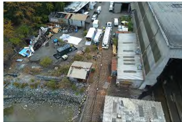
Oil removal operations from UAS overflight
