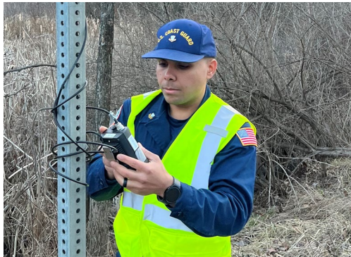
(Above) PO2 DeJesus-Vega performing maintenance on 1 of 8 RaeLink units networked for real-time air monitoring.
