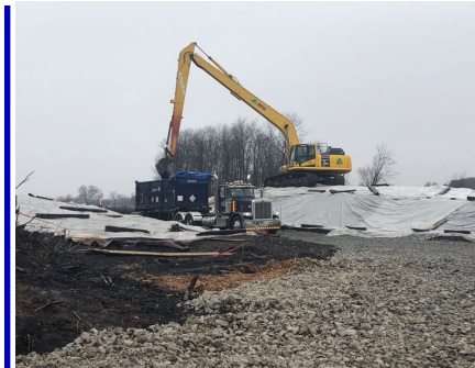
(Above) Removal of vinyl chloride contaminated soil for transport to disposal site.
