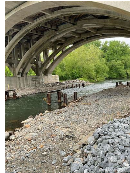
Narrow point under bridge of Interstate 78 that could be a potential area for boom deployment. Located next to boat launch area.
