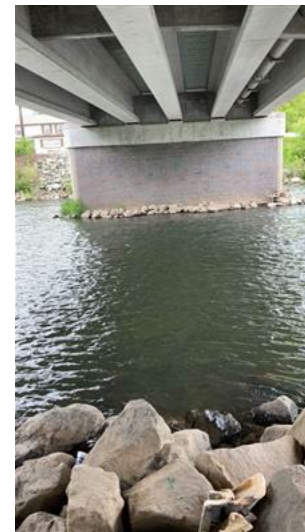
Location of potential anchor/float point under Wall Street Bridge located to the left of the control point.
