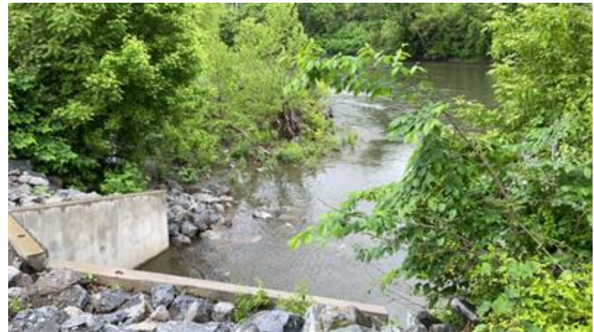
Stormwater outfalls near boat launch access that could serve as potential boom locations. There are also good anchorage points near control point.
